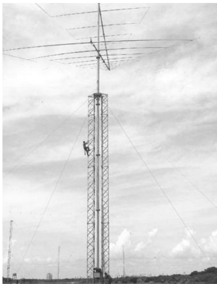
Adjusting a log periodic antenna at the Cape Canaveral receiver site.
